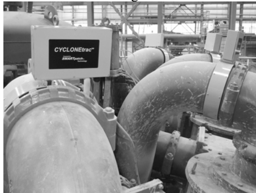
Figure 9: Oversize detection system on cyclone overflow
