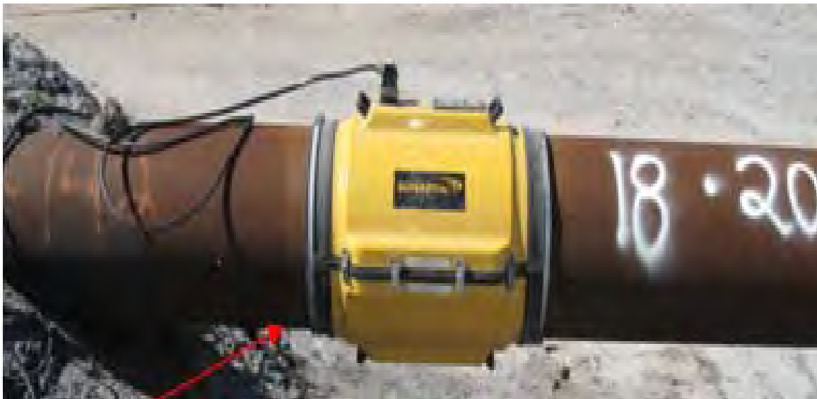
Figure 4 Field Installation at FCO
