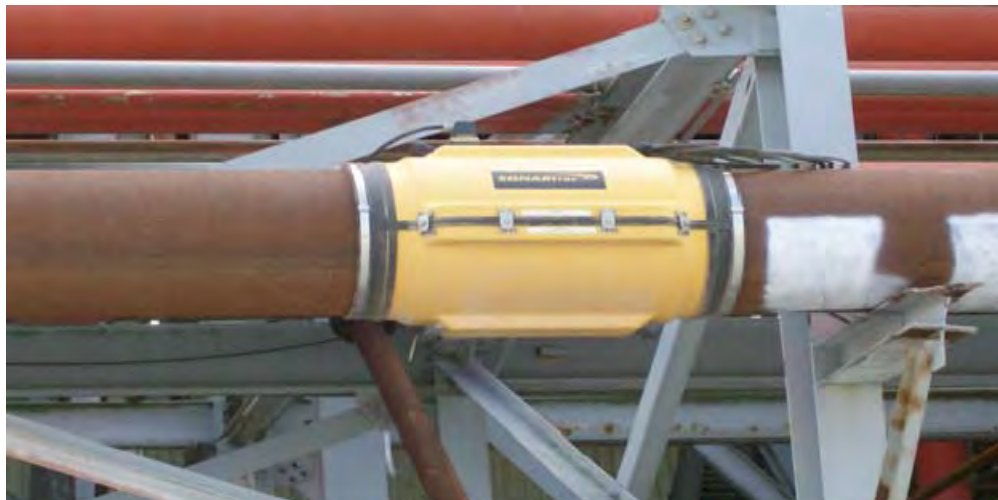
Figure 6 ONA Unit Current Installation
