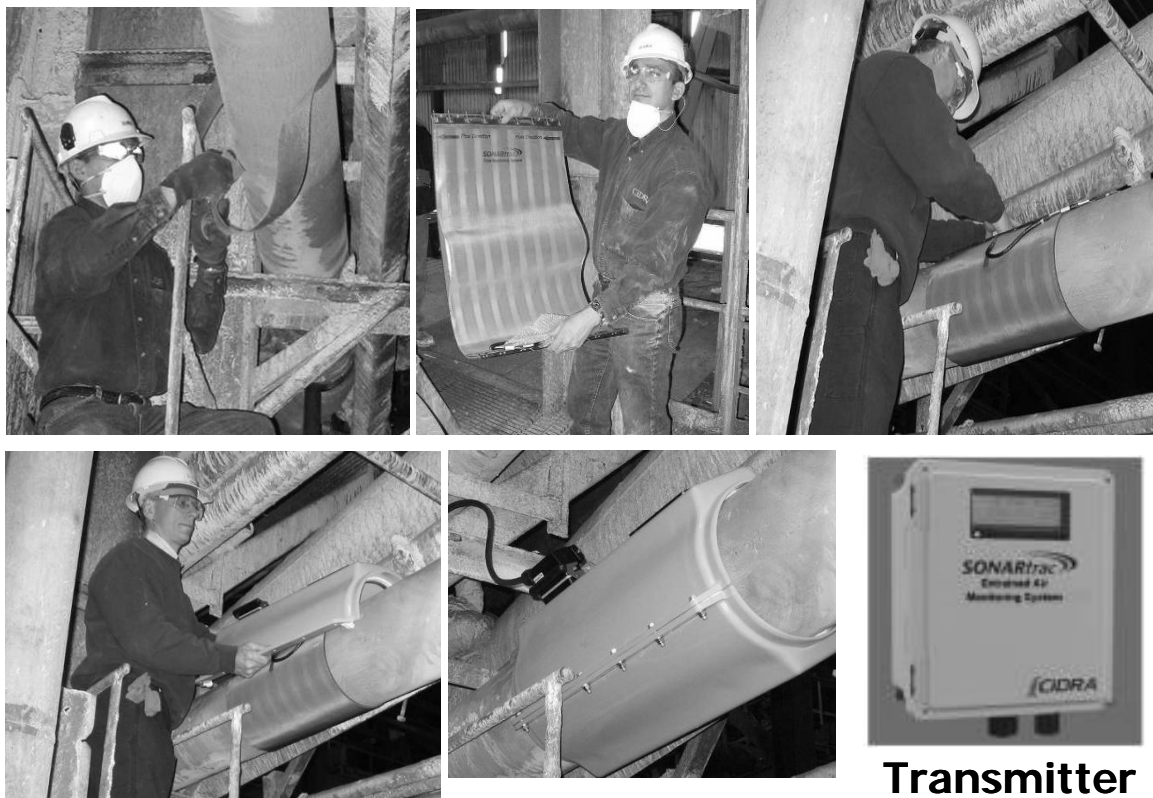
Figure 7 Installation procedure from (top-left) pipe preparation through cleaning and light sanding of pipe to (top-middle and top-right) mounting of the flexible, lightweight sensor band to (bottom-left) installation of this sensor cover and to (bottom-middle and bottom-right) connection of sensor cover to transmitter via water tight cable
