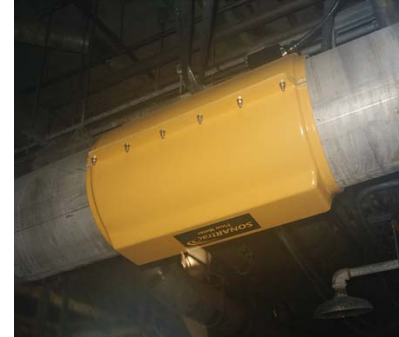
SONARtrac Meter installed On Basis Weight Line
