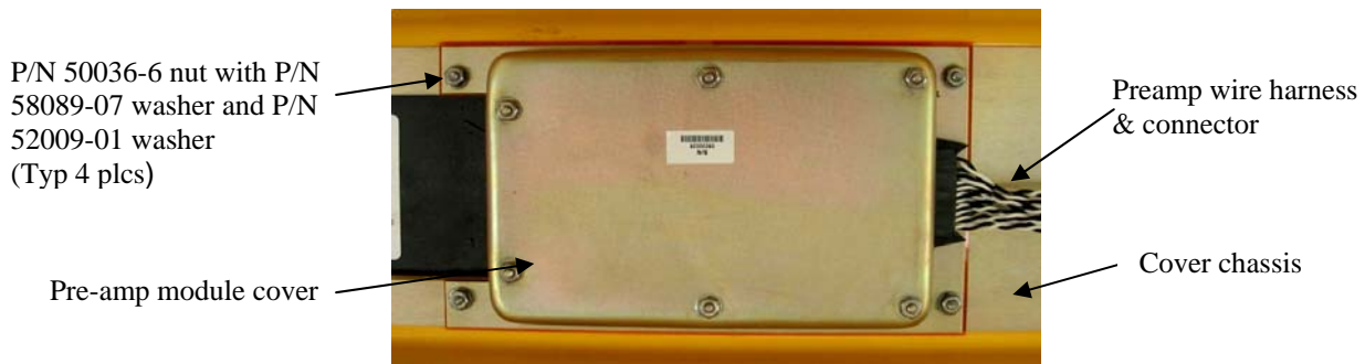
Figure 1 Pre-amplifier Module Installed In Sensor Cover
