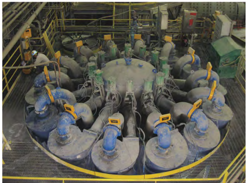
Figure 4—CYCLONetrac installed on hydrocyclone battery 8.
