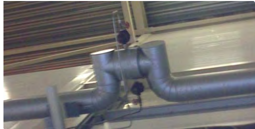
Figure 7 An example of an installation gone wrong.
