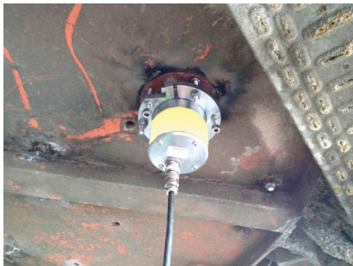
Figure 11: Installed sensor at precast plant
